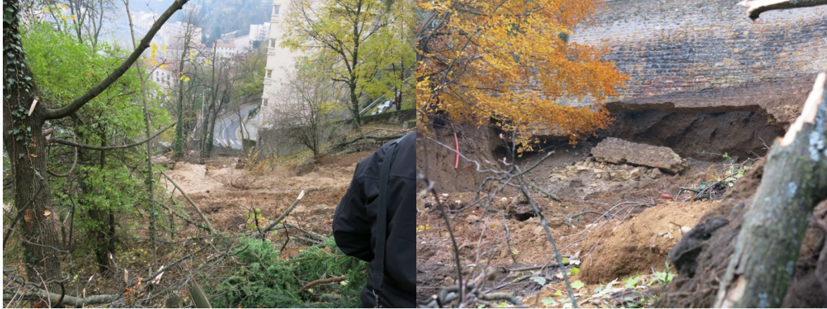
Fig.1. 2 pictures of the Lyon's landslide
